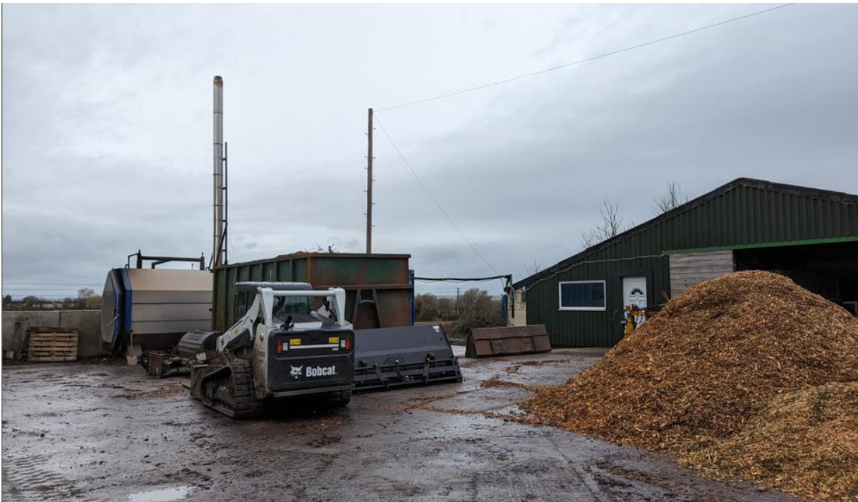
Photo taken on site of the boiler with the recently installed 6m high flue (and control room) and drying containers with the former piggery on the right
